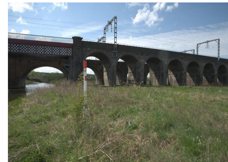
Fig 49 The proposed main path would utilise the second and third arches from the riverbank.
