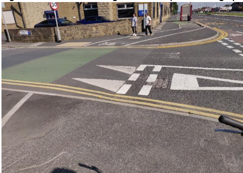
Figure 4-9 - Raised crossing in Bradford (WSP Photograph)
